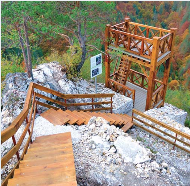
The Late Antique and Middle Ages Fortress 'Kaleta' near Koshnitsa village after the conservation works
