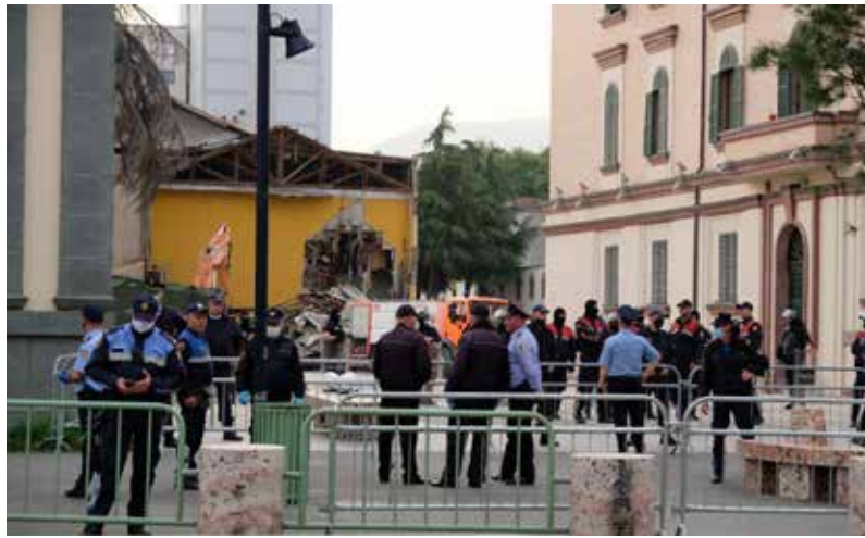
During the demolition of the National Theatre (photos by the Alliance for the Protection of the Theatre)
