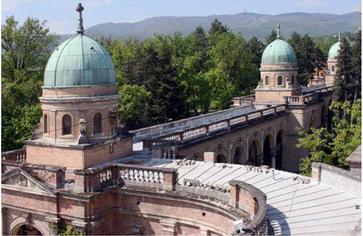
The damage to the roof of the Complex
