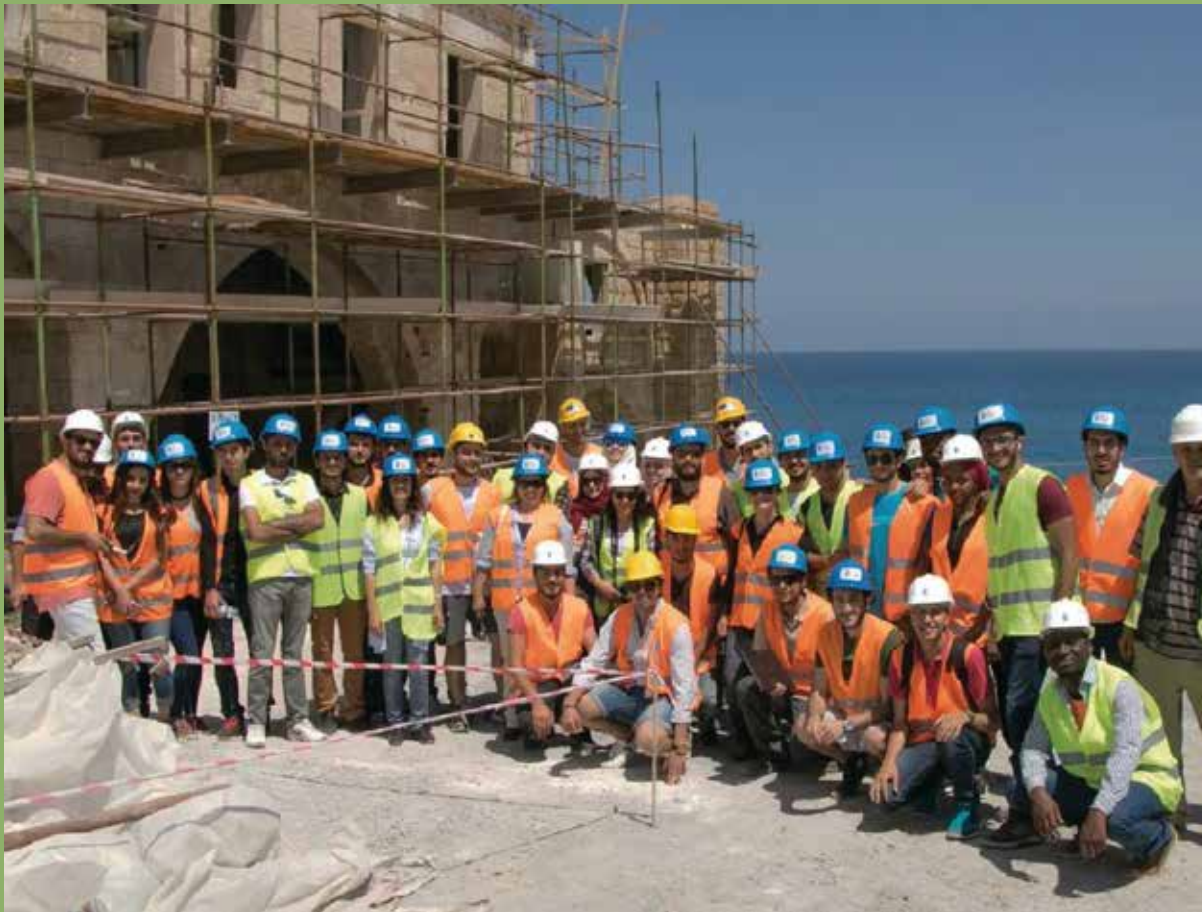
A restoration crew of the Technical Committee on Cultural Heritage (TCCH), Cyprus (photo courtesy of TCCH)
